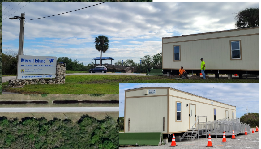
Left and above: Site preparations are underway for the Refuge's new Community Conservation Education Center which will be located off the northwest end of the existing Visitor Center parking area. The area is closed to visitors during this time. A temporary, accessible (ramp on south side) visitor contact station has been located at the west entrance to the MINWR with a "front desk" for providing maps, passes and information. Nature's Treasures Gift Shop, run by MIWA, will have retail items for sale there also.
